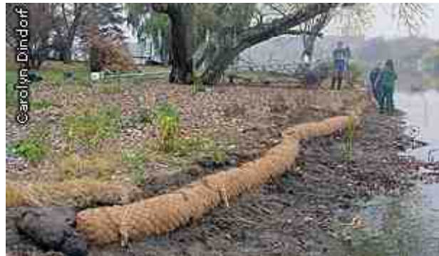
A coir log stabilizes an undercut bank with deep-rooted native species planted above. Source: Minnesota DNR https://www.dnr.state.mn.us/rys/sl/shoreline.html
