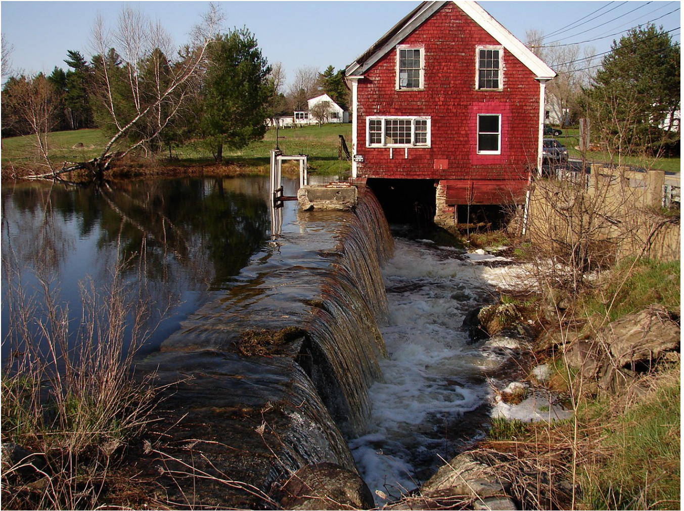
Illustration 2: This is not a flood event. This is routine over topping of the dam which is to be expected when the lake level is maintained at the Normal High Water Mark of the dam. Note the gate is wide open; total estimated flow is approximately 100 cfs. Photograph by George Fergusson April 30, 2008
