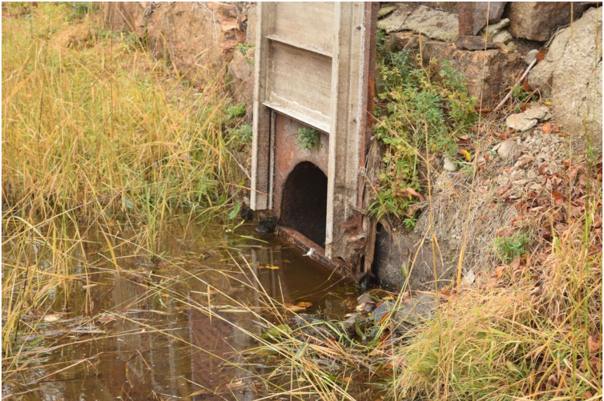
Illustration 1: Photograph of the Clary Dam gate showing the obstruction on the bottom. Photograph by George Fergusson 09 October 2017
